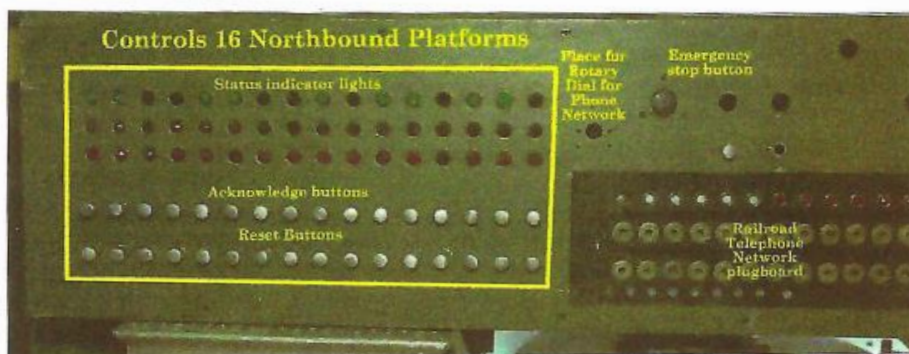
Train Directors Console also has the interface to the Railroad Telephone network (right side of panel).
